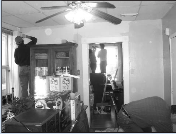
Above: Beginning in December 2007, Lowe's volunteers donated their time and supplies to make significant repairs to the Transitional Living Program house, the Emergency Shelter and the Kingshighway Head Start Center.
